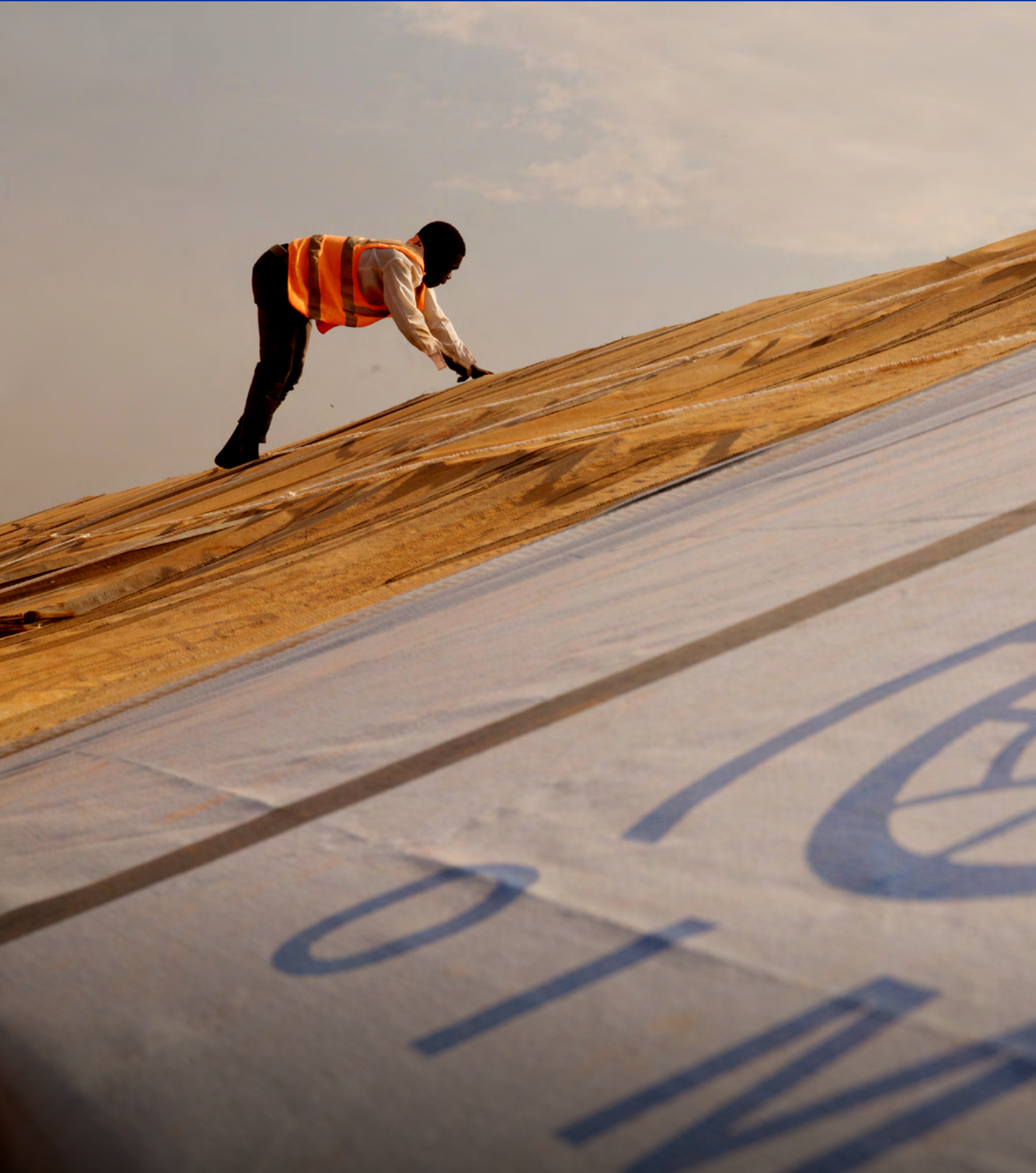
The Emergency Shelter team fixes a roof at Wau POC Camp. © IOM South Sudan 2020
